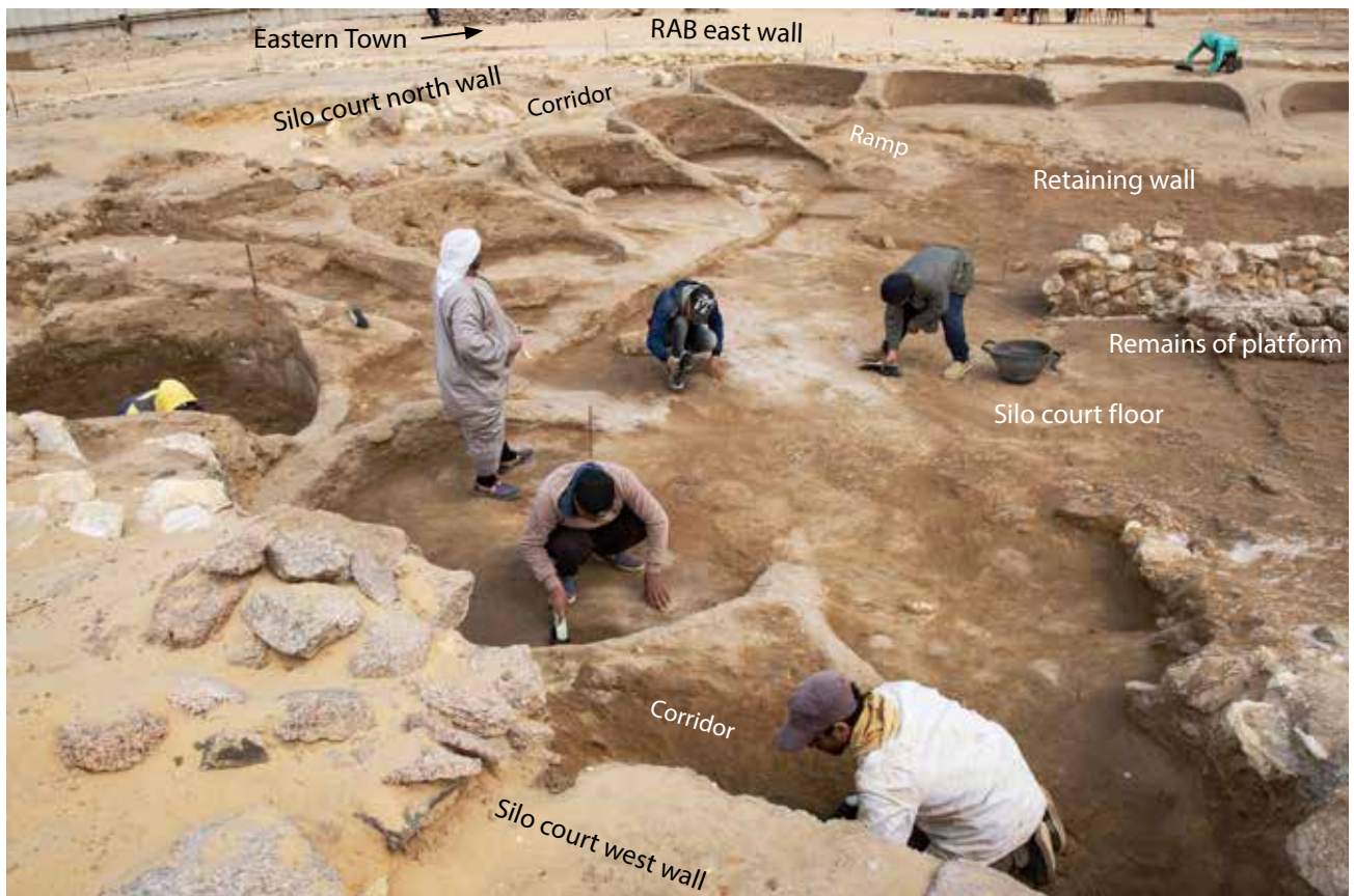
Below: The silo court on March 22, 2023. Workers clear the court floor and silos on the west side. View to the east.
